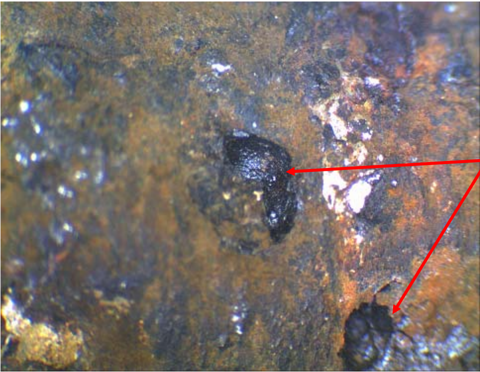
Kings crux bolt, significant corrosion damage.
